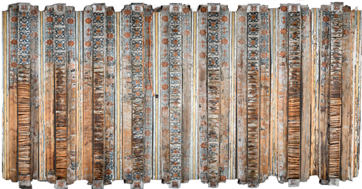
Fig. 5. Photogrammetry image of the ceiling before the intervention. It is possible to observe the three face-sides of the beams. Note the blue color tone variations between the beams, including at beam-face that is not exposed to light. (Photogrammetry & imaging: Misiones Coloniales de Chihuahua A.C., Montes Treviso F., 2024).
